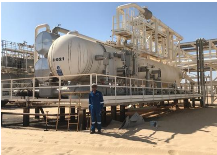
Figure 1. Low Pressure Production Separator C-021 (Personal visit)
